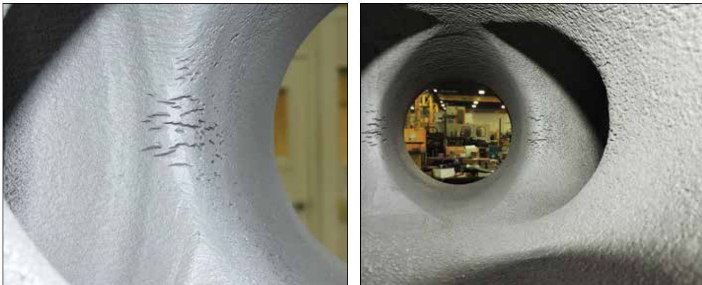
FIGURES 1 (LEFT) AND 2: Long-term, severe cavitation can cause surface pitting on a module crossbore and reduce the module's fatigue life. Over time, cavitation can lead to expensive maintenance issues and a potentially catastrophic failure.
