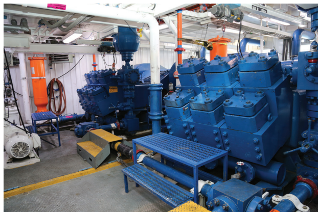
The mud system for Rig 90 features three Gardner Denver PZ-2400 pumps. (Source: AKITA Drilling)
